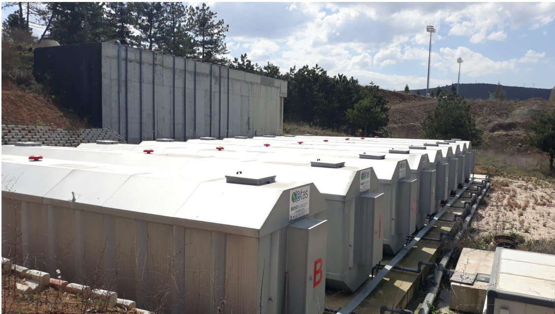
WWT Units, six packs total 900 m 3 /day Wastewater Treatment
